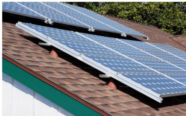
BAPV Roof-Mounted Photovoltaic System
